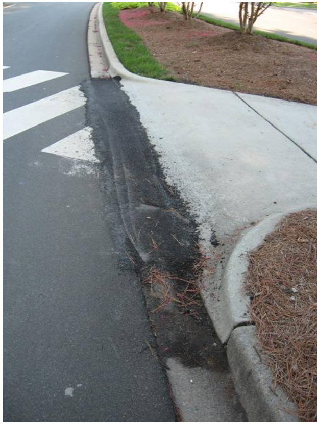
Asphalt Fill in Lip on American Tobacco Trail at Woodcroft Parkway
